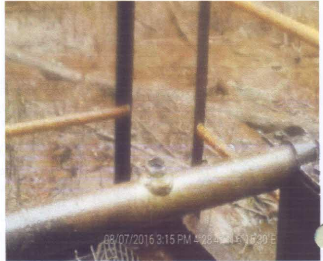
Figure 2: Affected 4" Gas line
